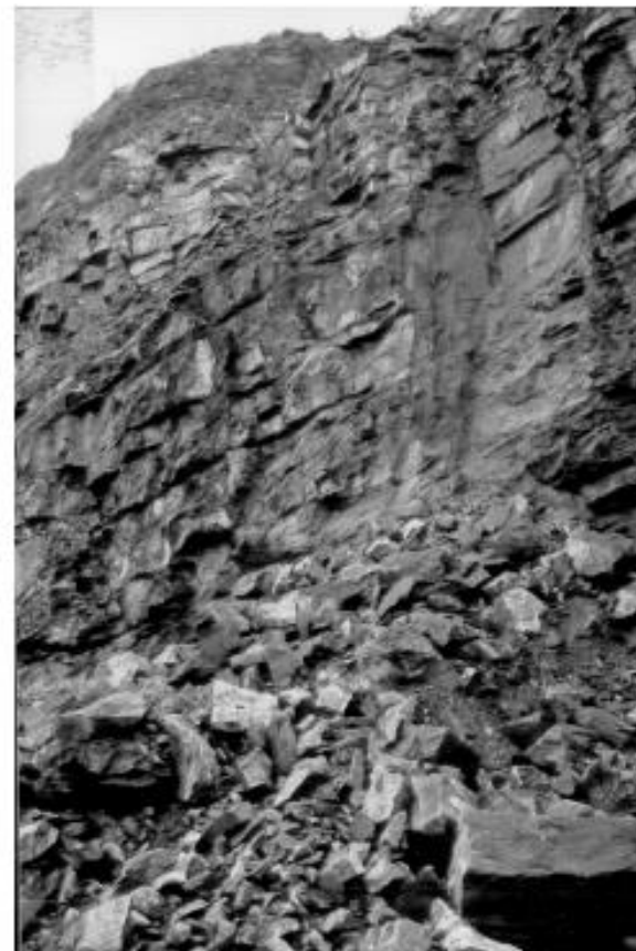
Fig. 23. Structurally controlled failure in the face of a steep bench in a heavily jointed rock mass.
